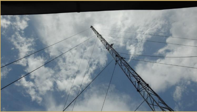
Radio and TV Transmission Antenna
